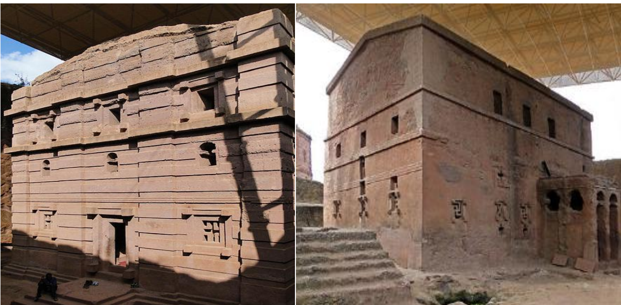
Figure 11: Level of Damage in Bete Amanuel (House of Emmanuel) & Bete Maryam (House of Mary)
