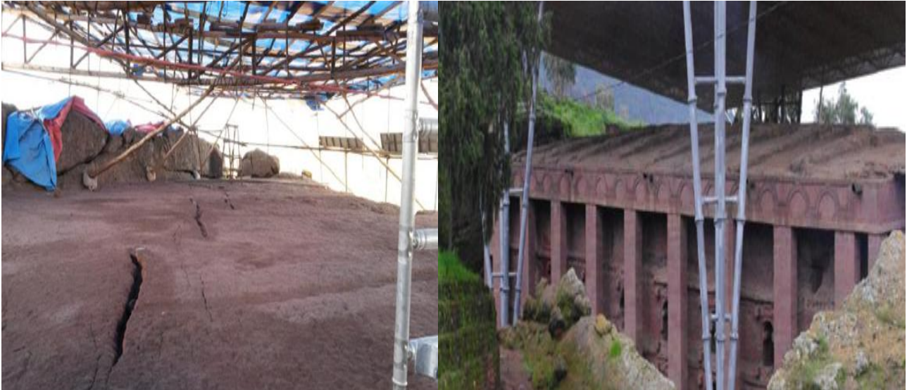
Figure 4: Crack on Bete Gabrel Roof (House of Gabriel Raphael) – Bete Medhane Alem (House of the Savior of the World)
