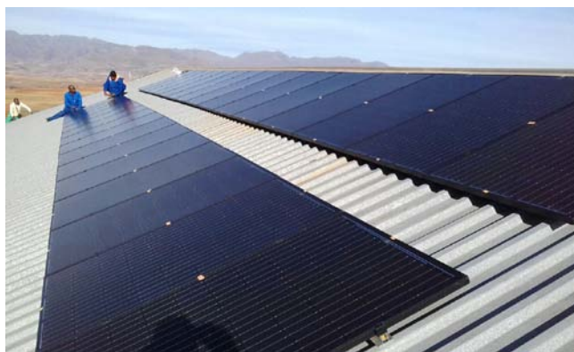
Figure 15. PV Array installed at Malealea Lodge in August 2016.
