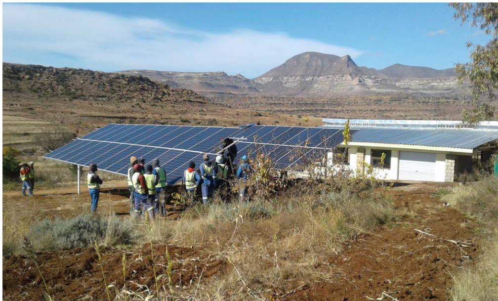
Figure 8. New Solar Lab and 16.5kW Solar Farm completed in 2019 on BBCDC campus. Balance of system includes a 10KVA sine wave inverter (230V AC) and a 20kWh battery storage.
